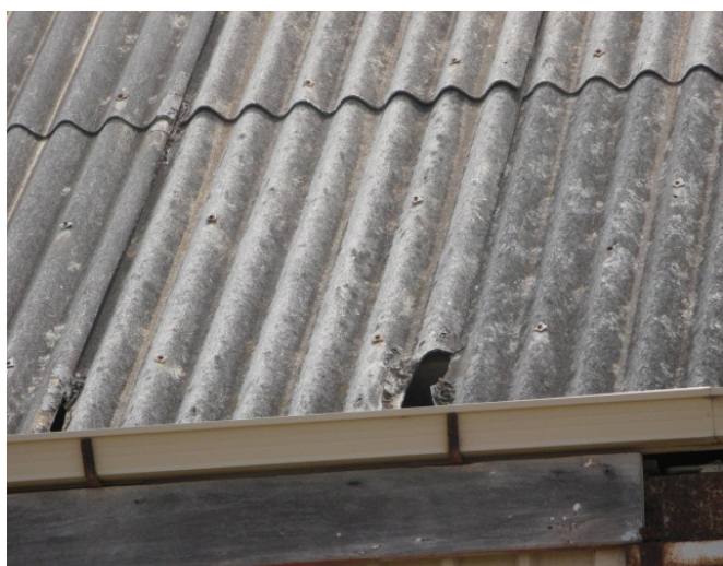
Photo 7. ACM roof breakages
