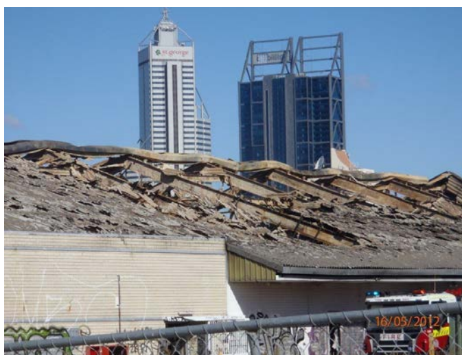
Photo 8. Shattered ACM roof resulting from fire
